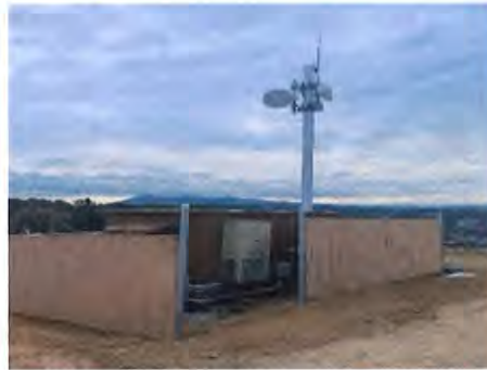
Skyview Terrace microwave site.
