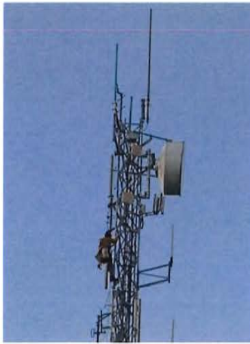
Microwave work at the Dollar Hill Site
