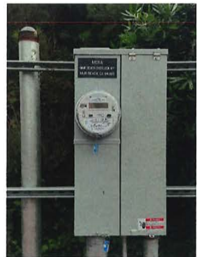
PG&E meter installed at Muir Beach Site.
